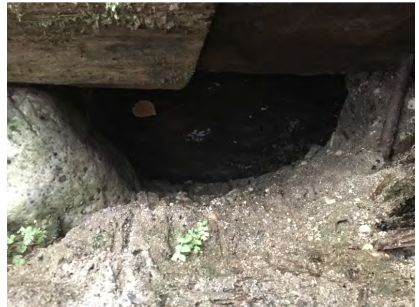
Top layer of stringer have conk noted
